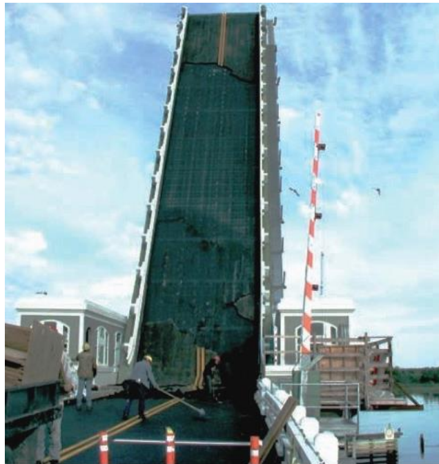
Figure 131 Wearing surface failure of the Lewis and Clark Bridge (Bottenberg 2010)
