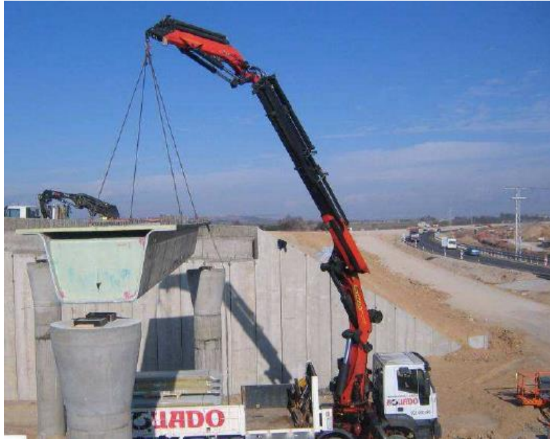
Figure 120 One of the beams lifted in place by crane truck (Burgos Muniz 2012)
