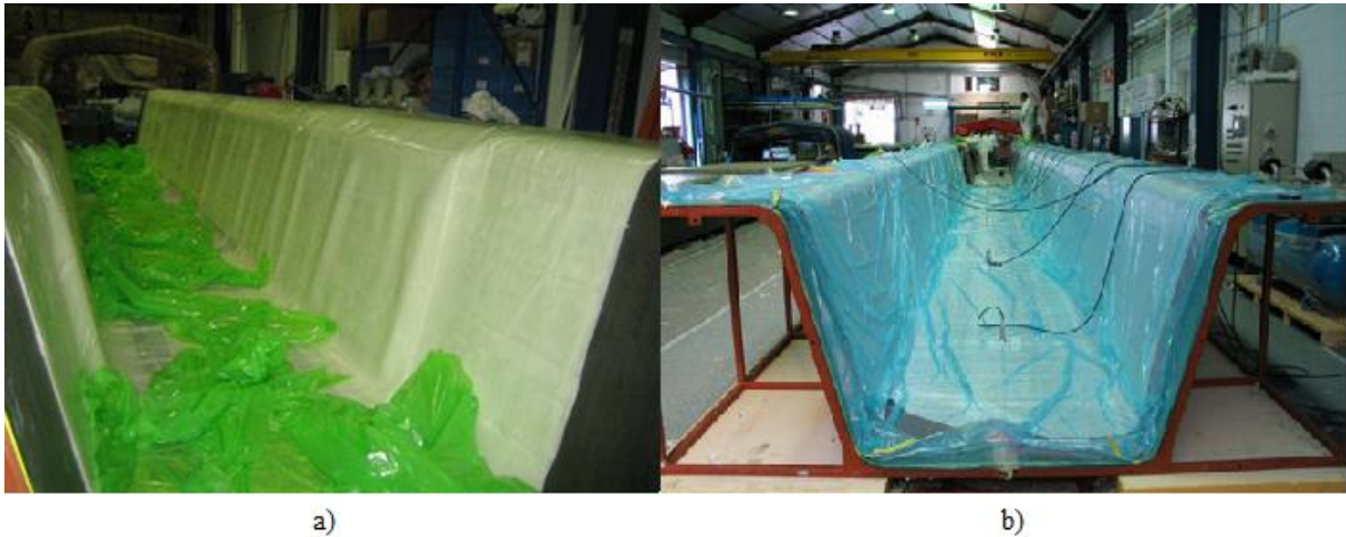
Figure 118 Manufacturing process a) Lamination (Burgos Muniz 2012) b) Vacuum bag preparation (Burgos Muniz 2012)
