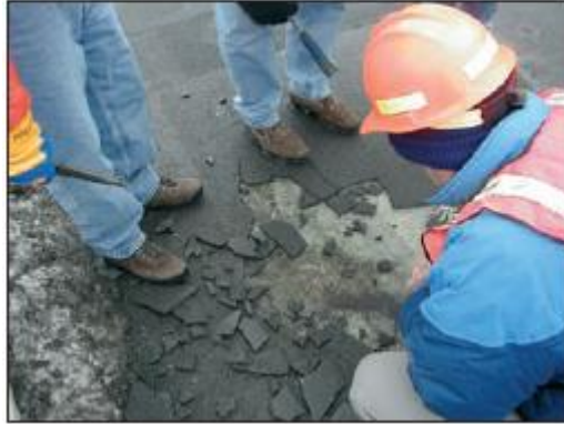
Figure 130 Wearing surface debonding due to thermal loads (O'Connor & Triandafilou 2010)
