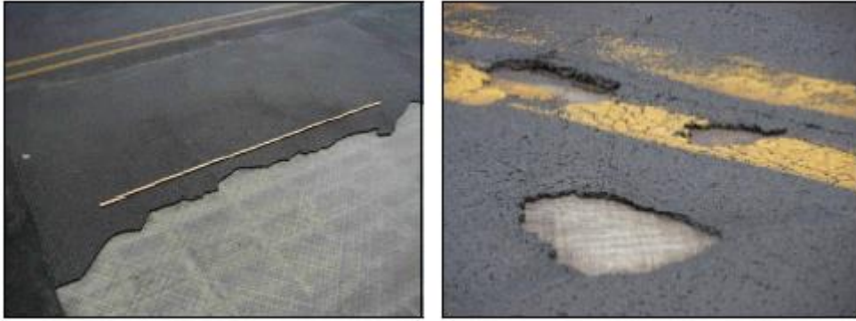
Figure 128 Wearing surface as deboning problem (O'Connor & Triandafilou 2009)
