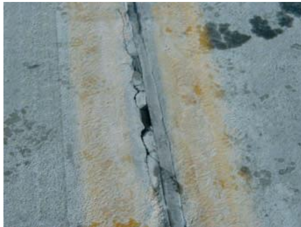
Figure 129 Cracking between FRP composite panels (O'Connor & Triandafilou 2010)
