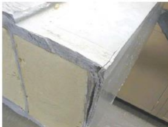
Figure 91 Void found in the face sheet of sandwich deck (Meyer 2006)
