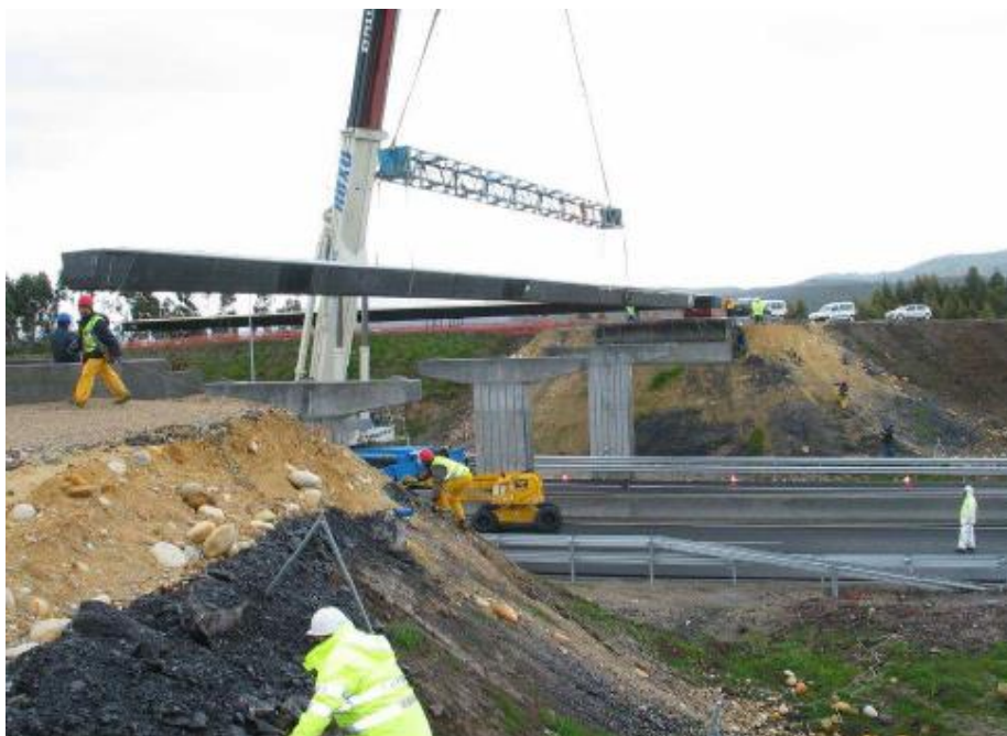
Figure 115 Using crane to install the girders of the Asturias Bridge (Areiza Hurtado 2012)
