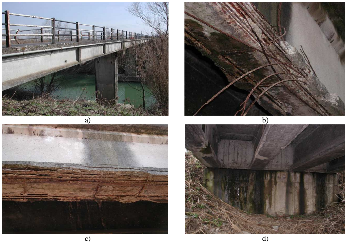
Figure 7: Visual inspection on the bridge: a) General view; b) Corrosion of pre-stressing wires; c) Concrete spalling and reinforcement corrosion; d) Degradation of concrete surfaces.
