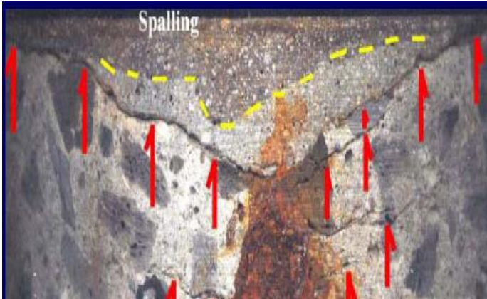
Figure 29 Delamination provoked by the corrosion of reinforcement [7]
