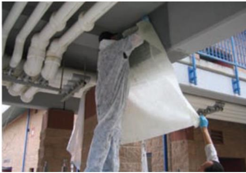
Figure 15 Application of the Prepreg based on glass fibers in order to increase shear capacity of the beam
