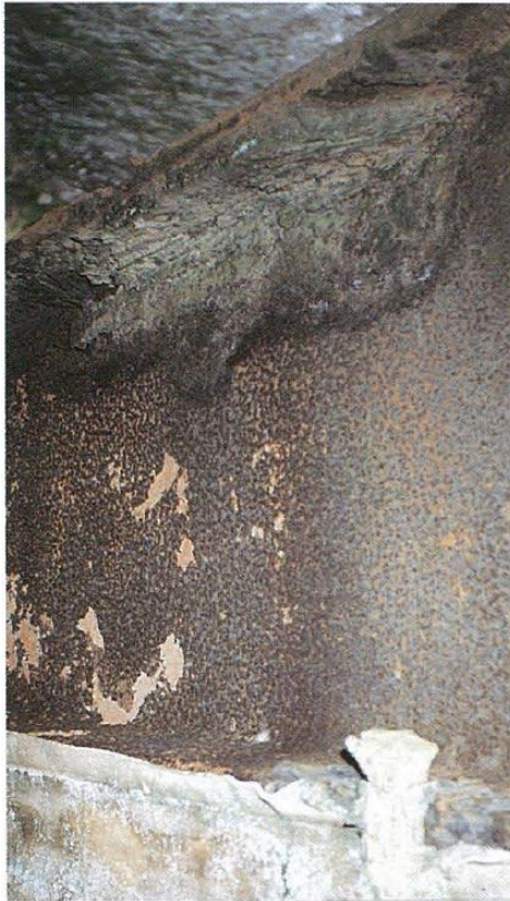
Figure 5 Damp patch caused by accumulated rust and debris [1]
