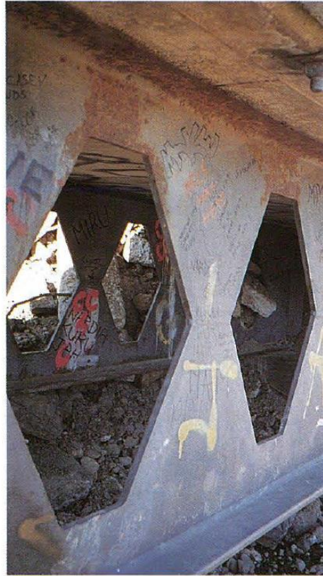
Figure 6 Effect of rain washing: removal of marine salts by rain washing has kept bottom of outer beam corrosion-free for 14 years (red lead/MIO alkyd system) [1]
