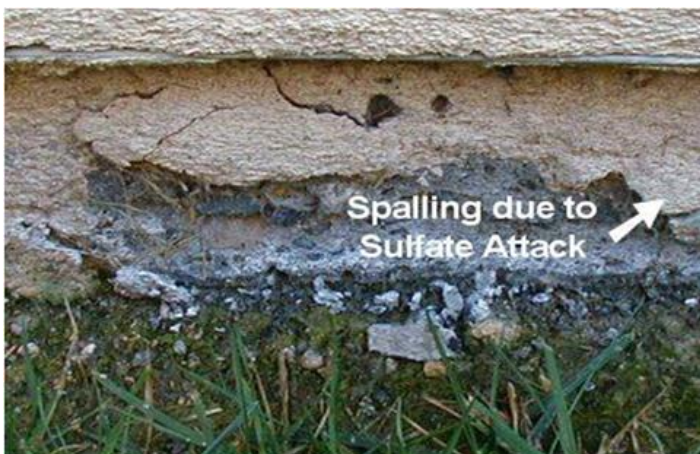
Figure 37 Spalling caused by sulphate attack [11]
