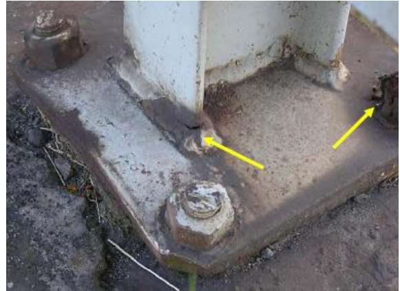
Figure 17 Weld crack at the base and corrosion of nut [6]
