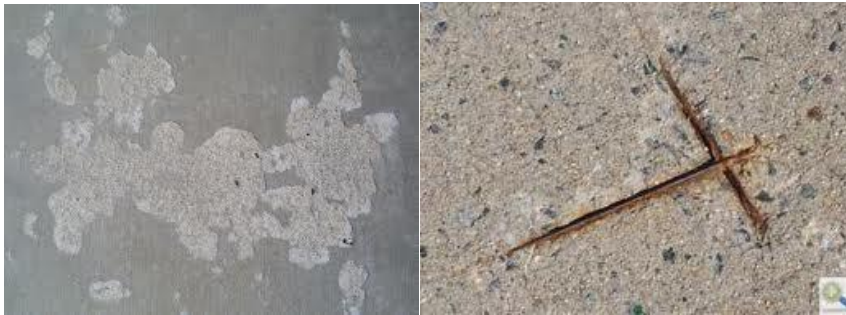
Figure 22 Example of scaling in concrete
