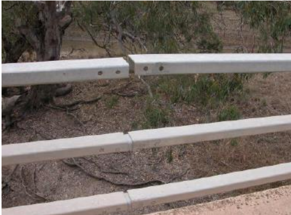
Figure 16 Rail connector missing [6]
