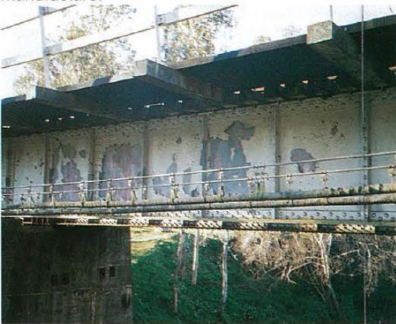
Figure 3 Incompatible coatings (alkyd paint over zinc-rich) [1]
