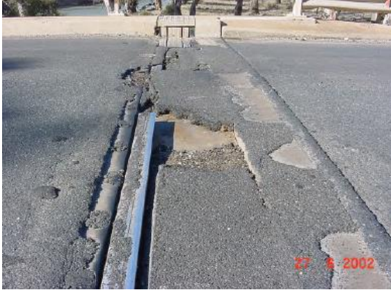
Figure 10 Joint in poor condition [6]
