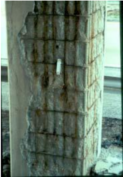
Figure 30 Corrosion damage to concrete bridge pier [9]
