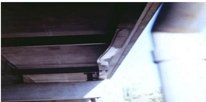
Figure 9 Accident damage in a steel girder caused by an over-height vehicle [4]
