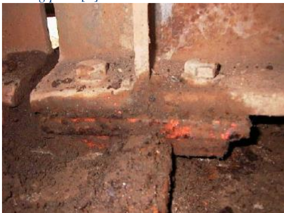
Figure 20 Significant corrosion with pitting [6]
