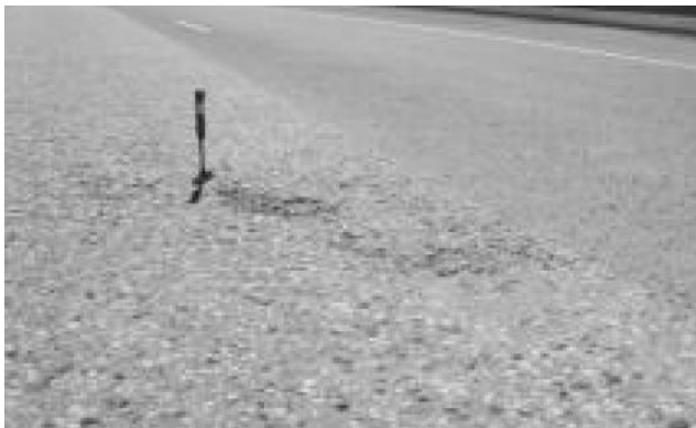
Figure 34 Example of abrasion damage [7]
