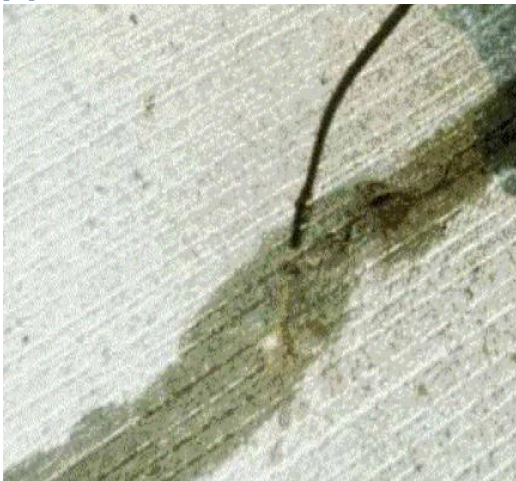
Figure 26 Example of flexural cracks [7]
