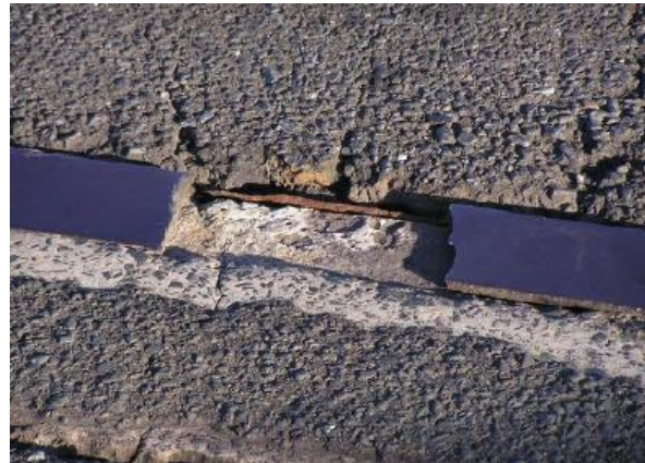
Figure 13 Loose and broken protection angle [6]
