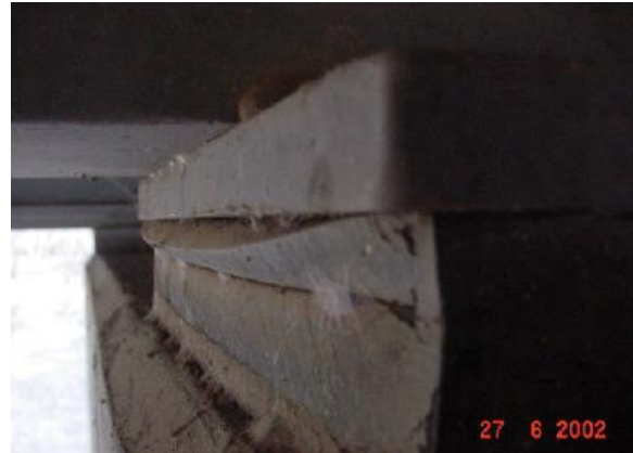
Figure 19 Significant bulging of bearing pad [6]
