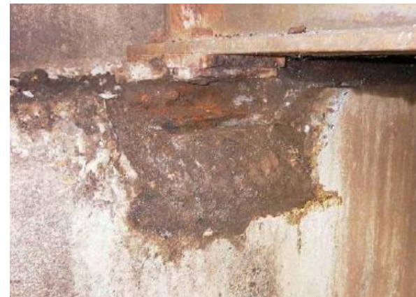
Figure 21 Significant loss of support under the bearing [6]
