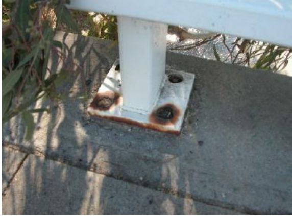
Figure 14 All the nuts and parts of bolts completely corroded off [6]
