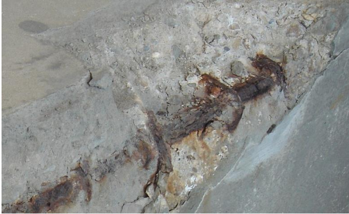
Figure 38 The effects of carbonation on concrete (photo by MADe)
