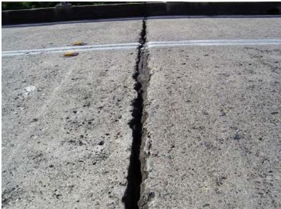
Figure 12 Seal has failed leading to extensive water leakage through the joint [6]
