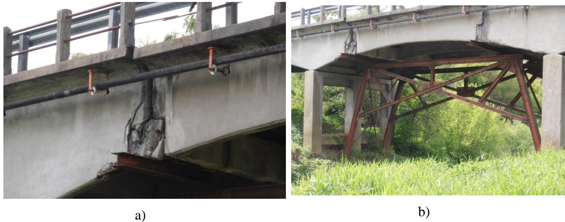
Figure 3 Bridge on a canal at Bientina (Pisa), Italy – Road S.R.T 439 km 51: a) Breakage of the internal hinge of the Gerber beam; b) Provisional support structure built by the Administration
