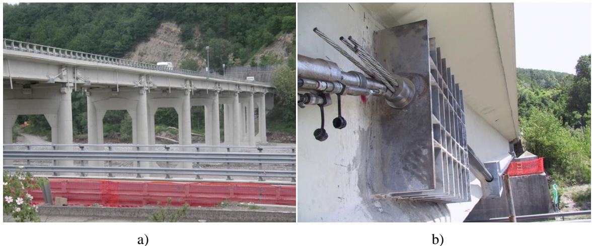
Figure 15 Bridge on the Taro River at Solignano (Parma), Italy – Road S.S. 308 km 11+850: a) View of the bridge; b) Detail of an external cable anchoring device made of steel. The project included reinforcement of the bridge's piers, deck, and longitudinal beams. The intervention was performed with one-way traffic open during 2003 - 2004).
