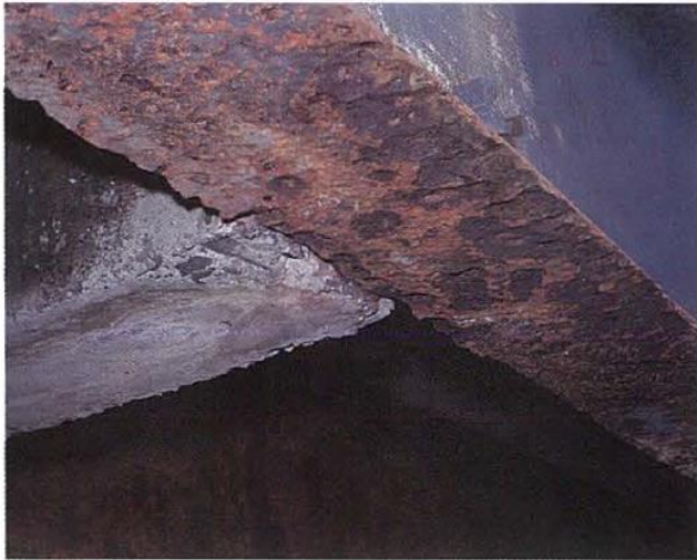
Figure 1 Loss of section, severe pitting due to condensation and concentration of salts on bottom flange (and lack of maintenance) [1]
