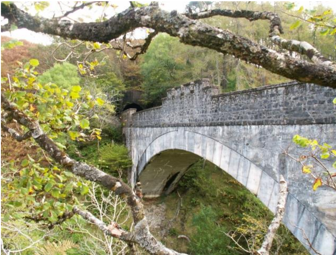
Figure 26 Borrodale Viaduct, Scotland, UK, built in unreinforced concrete (photo by Jim Bain)
