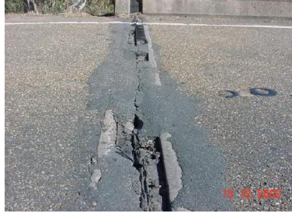
Figure 11 Joint in poor condition [6]
