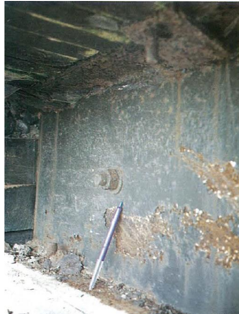
Figure 2 Coating failure caused by inadequate primer [1]
