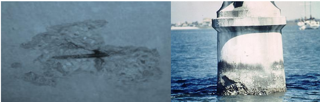
Figure 23 Example of spalls in concrete
