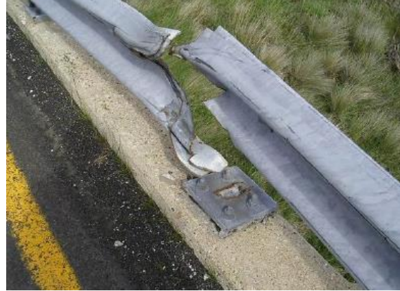
Figure 15 Badly damaged metal railing with missing post and torn guard fence rail [6]
