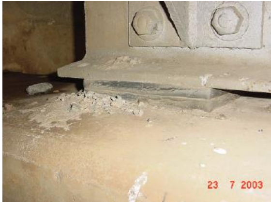
Figure 18 Significant splitting and bulging of bearing pads [6]
