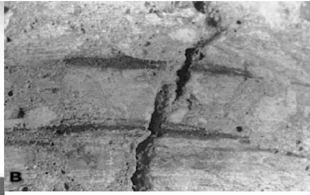
Figure 25 Example of drying shrinkage cracks [7]
