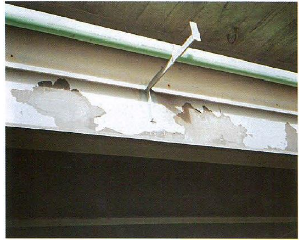
Figure 4 Loss of adhesion (inadequate surface preparation) [1]
