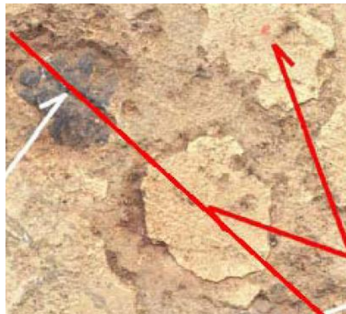
Figure 35 Example of mortar flaking damage [7]
